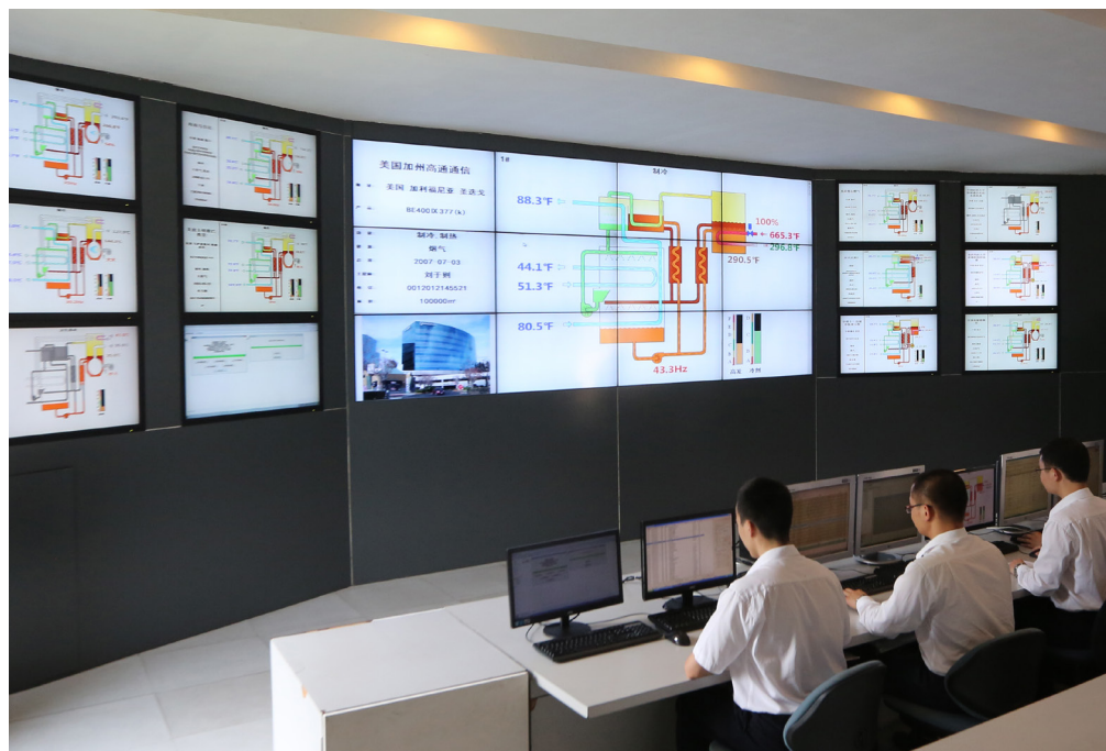
Global internet monitoring system for BROAD non-electric chillers. It has been operating since 1996, known as the originator of "internet +"
