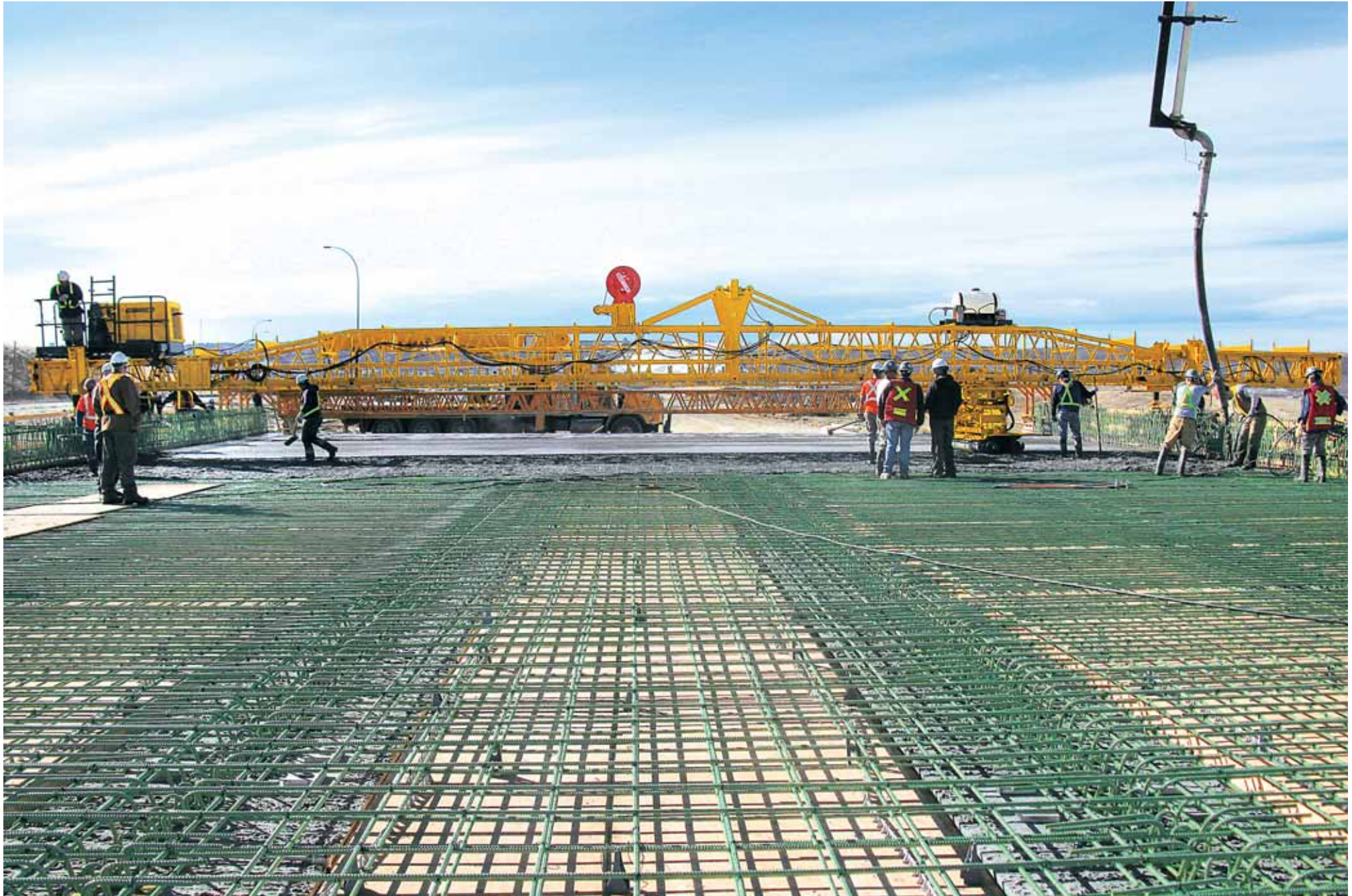
A C-450 with transitional framework finishes a bridge deck on a skew with its double-cylinder carriage and a four inch (102 mm) crown built-in with a power transition adjuster (PTA).
