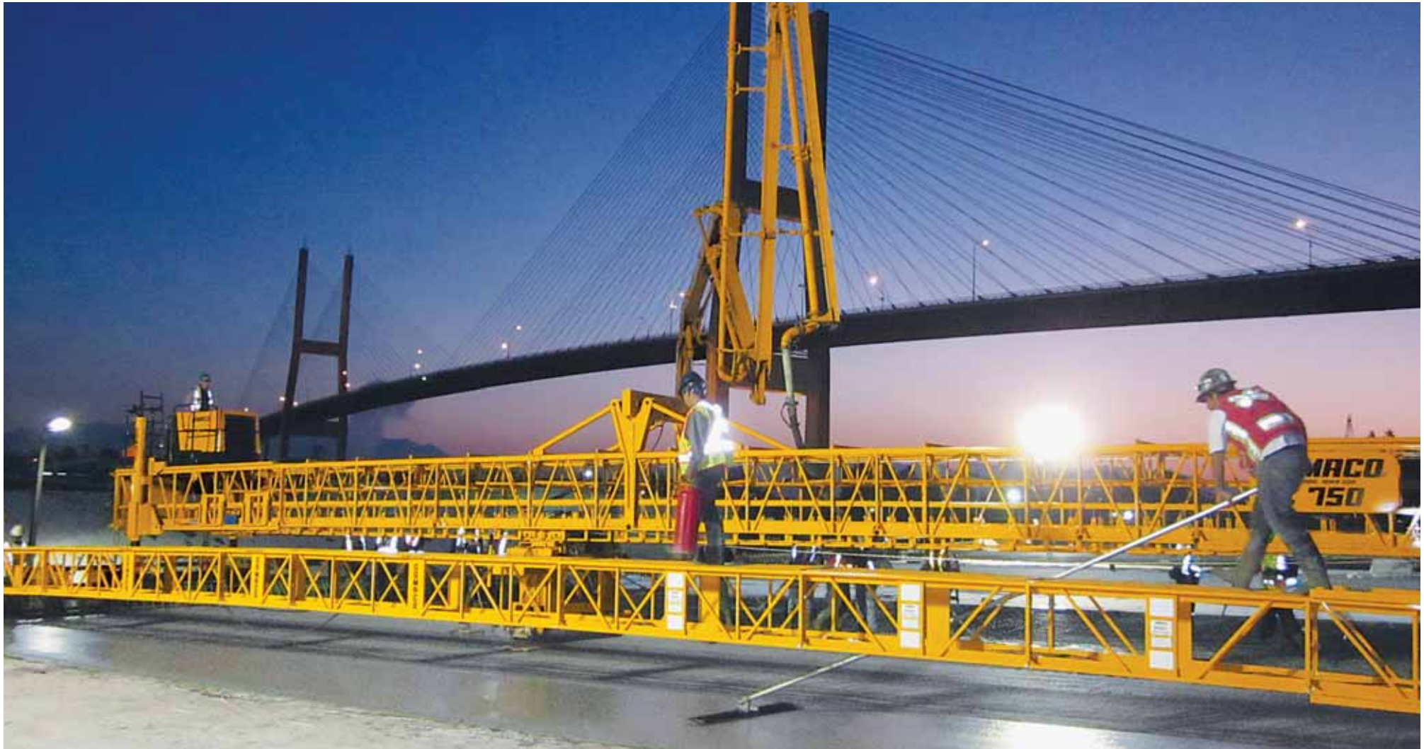
The GOMACO C-750 with a power transition adjuster (PTA) is finishing a bridge deck. It is followed by a powered Spanit® Work Bridge.
