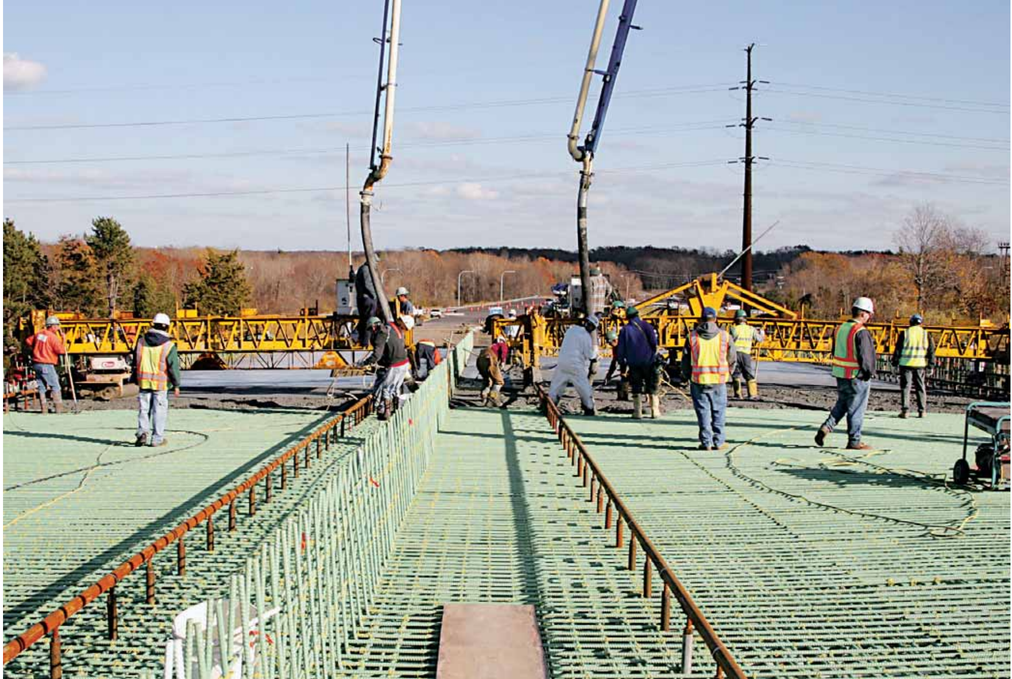
Two C-450s work side-by-side with two concrete pumper trucks to finish this bridge deck.
