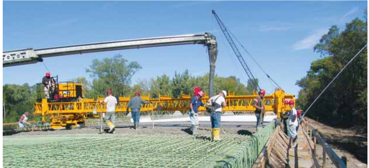
The C-450 finishes a 48 foot (14.63 m) wide bridge deck with a thickness of 20 inches (508 mm).
