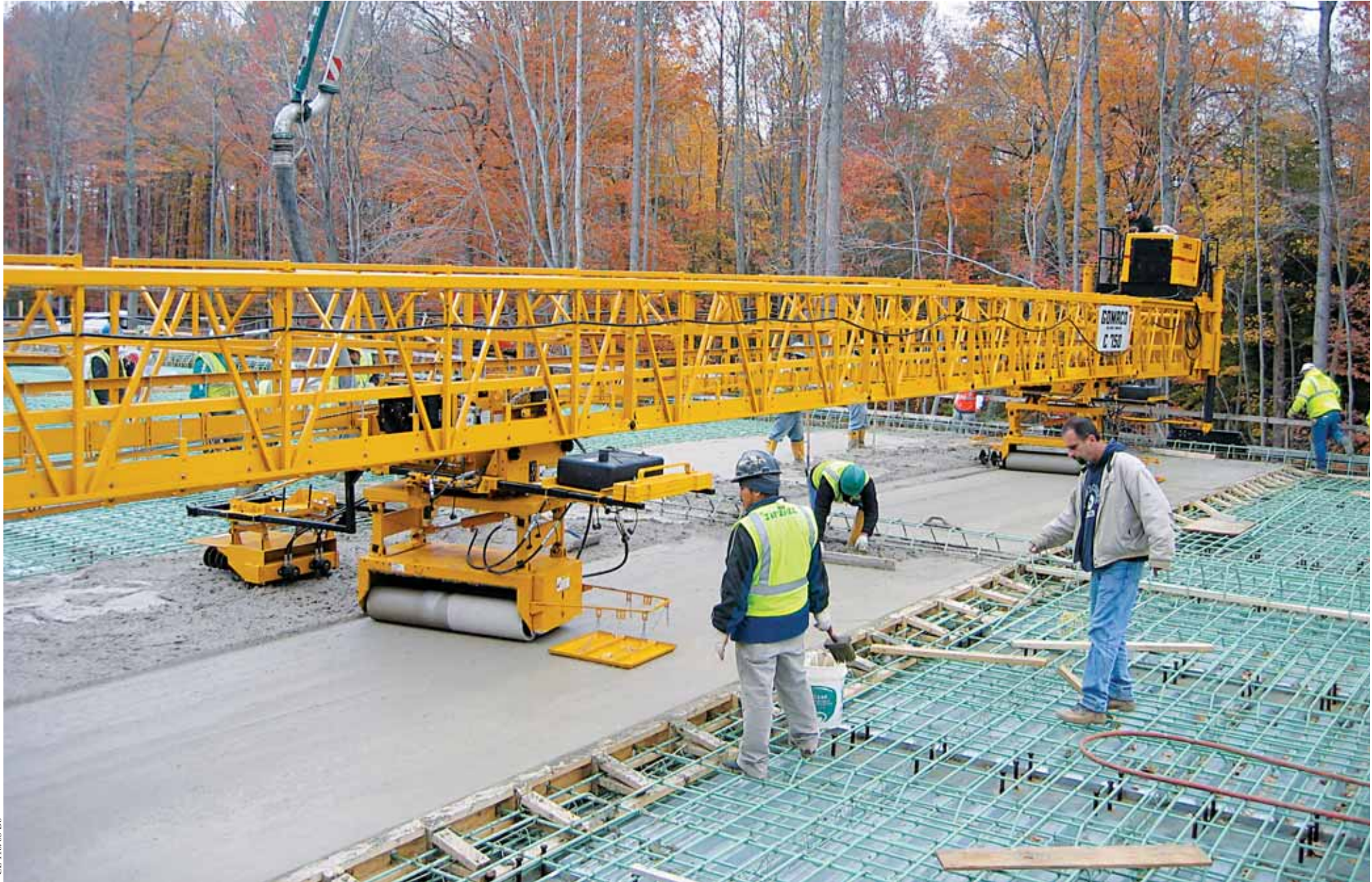
This GOMACO C-750 uses two, three-point finishing carriages for maximum efficiency to pave both sides of a bridge deck. The left carriage has the adjustable double augers and the right carriage has the standard augers, which operate ahead of the finishing cylinders.
