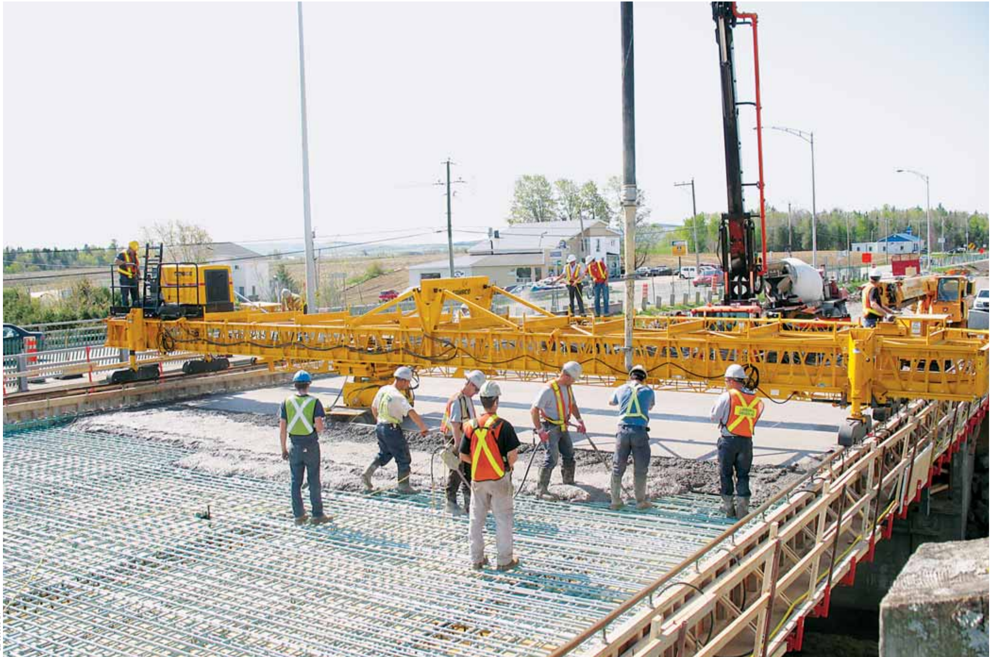
The C-450 with a PTA is finishing a 225 foot (68.58 m) long by 44.5 foot (13.56 m) wide bridge deck.
